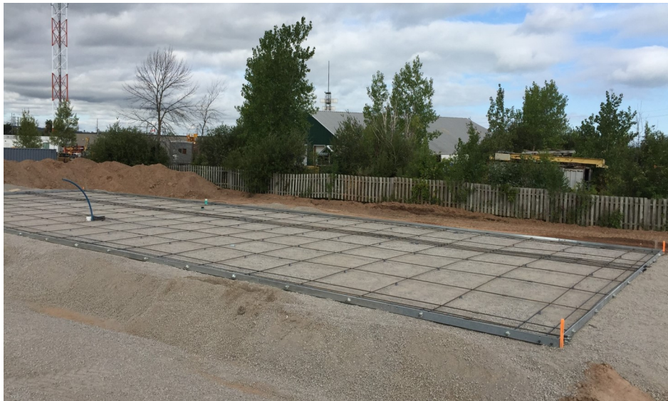
MK5 SERIES FOUNDATIONS ARE DESIGNED AS A SUSPENDED SLAB, INVERTED, USING 150 GRADE HIGH-YIELD POST TENSION BAR UNDER COLUMN AND IN A STRUCTURAL SLAB GRID CREATING A 2-WAY REINFORCED CONCRETE AS A STRUCTURAL FOUNDATION SUPPORTING SUPER-STRUCTURE LOADS, ON GROUND.
